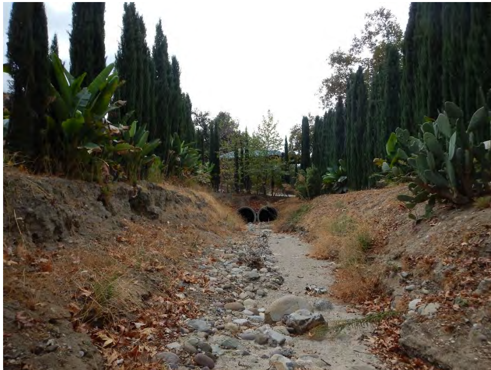
Photo 10 – View of the Live Oak Canyon Drainage where it becomes channelized and culverted through the active Saddle Club property, facing south.
